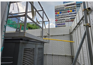
Generator noise barrier
