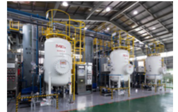
Refrigerant recycling and purification facility
