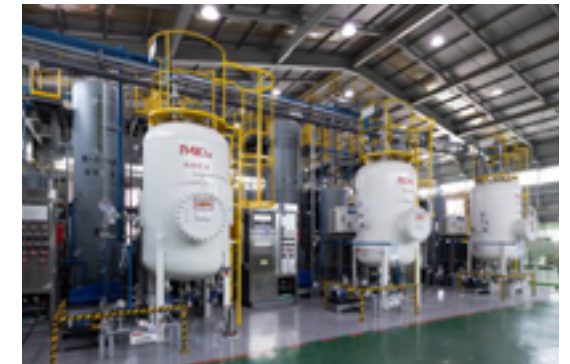
Refrigerant recycling and purification facility
