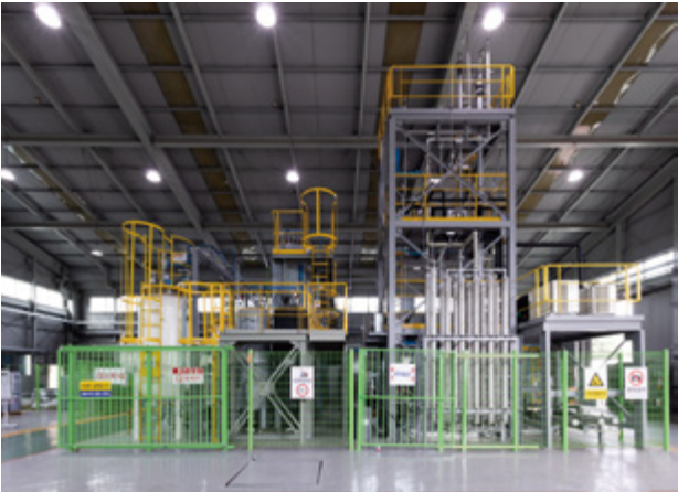
FINEXG Recycling Facility
