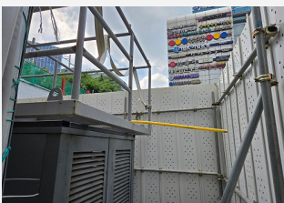
Generator noise barrier
