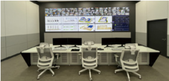
STELLA Control Room
